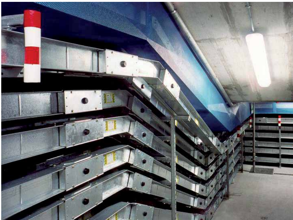
Example of high power distribution
